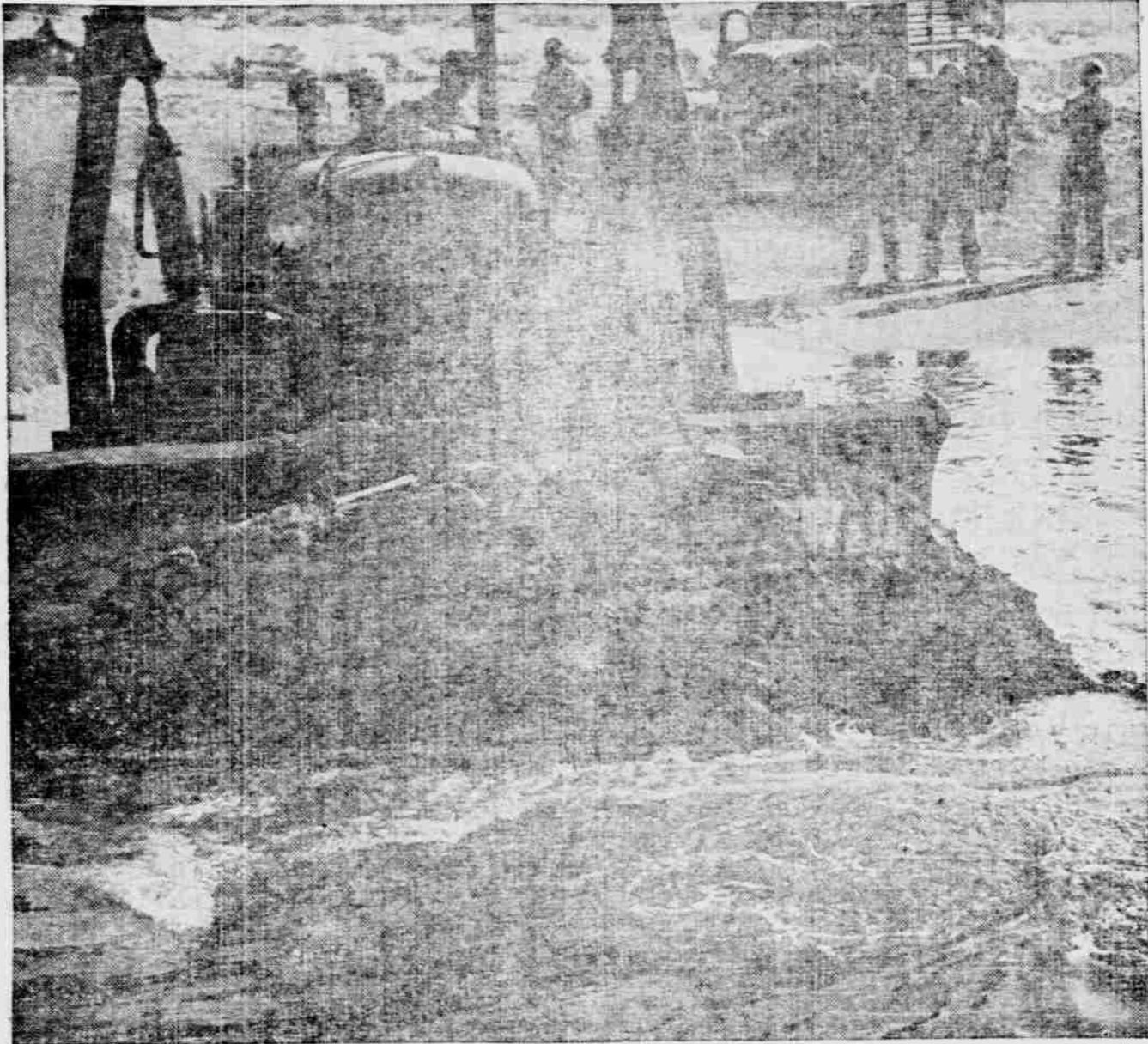
When the American Army moves it does things in the American way. At Pesto, Italy, 25 miles South of Naples the bulldozers moved in with the first waves of Lieut. Gen. Mark W. Clark's invading Fifth Army. Here is shown one of them building a road right down to the landing beach. The War Bonds you buy are helping build that road that is leading to Berlin and Tokio.
