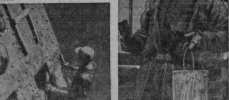
Painting this giant is an awesome job to this workman as he ponders how many pailsful it will take to "spot" paint the Quebec Bridge.
