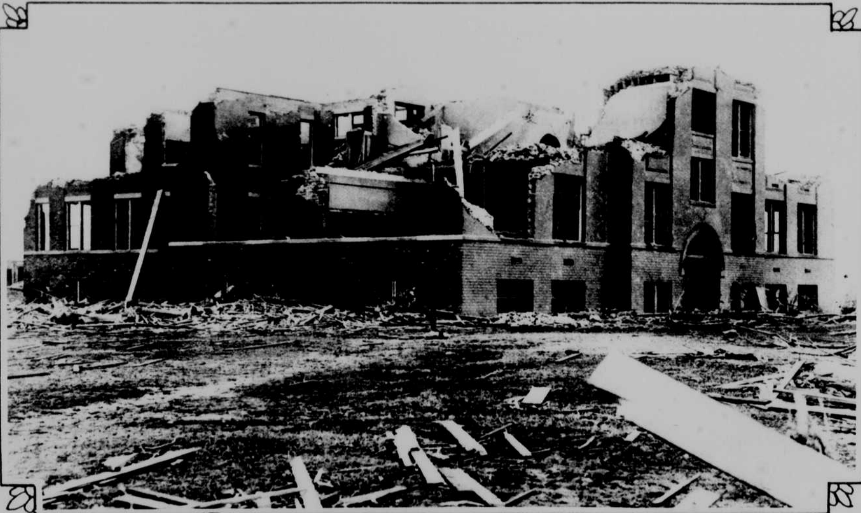
All that remained of the Longfellow School at Murphysboro, Ill., where a number of children were killed or burned to death in the wreck caused by the tornado. This Ill. town was the worst hit.
