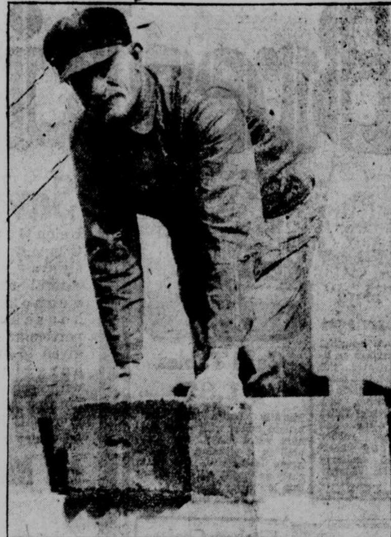
Fred Albers, who is declared to be one of the most experienced concrete men in Omaha, is busy as the proverbial beaver. He's called upon to do a lot of the "fancy stuff" in building the Ideal Firesafe Home walls and corners.
