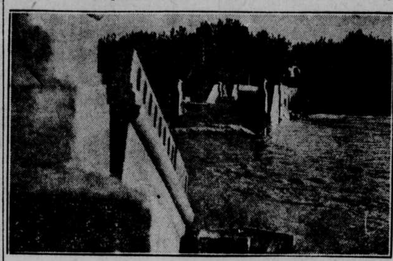
Here is the wreckage of the state bridge across the Republican river at Bartley, Neb., on the Lebanon road, which was swept out by high water.
