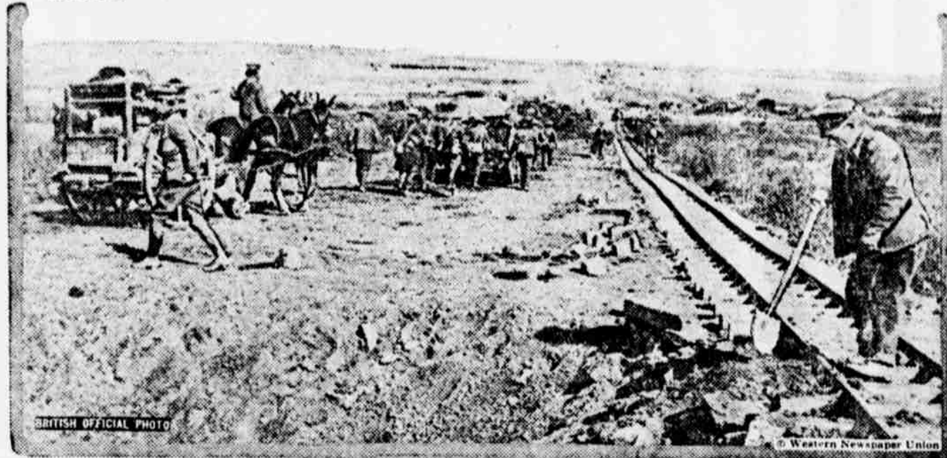
The reconstruction period is now sweeping over all of the battle-scarred area of France and the roads are being rebuilt. This photograph shows a scene on a road in the vicinity of Cambrai that was mined by the retreating Germans. The British constructed a light railway and a new road.
