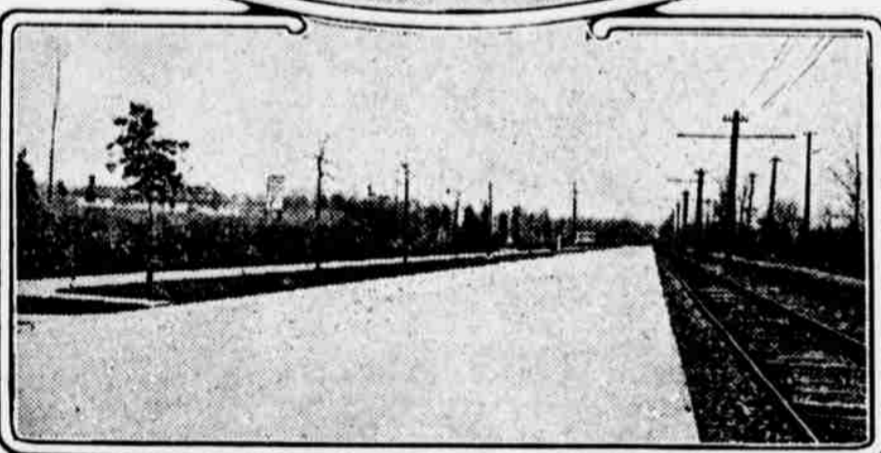
Construction of Concrete Road—Sand and Gravel Piled on Subgrade Ready for Use—Subgrade Prepared for Concrete Pavement—Road After Nearly Two Years' Service.
