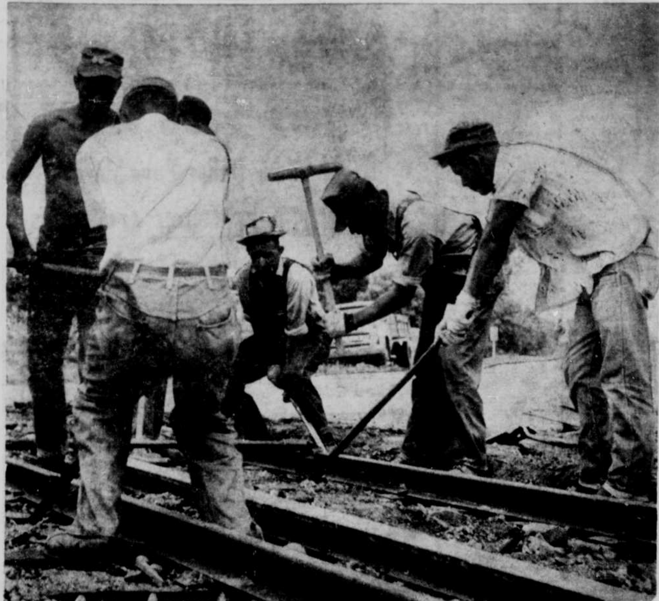
It's still tough, this working on the railroad business. The Burlington crew came to O'Neill to replace tracks across Highway 20 when the old road became too rough for automobile traffic. A state highway crew followed the work of the railroad and re-rolled the crossing after the old rails were torn away and new ones replaced.
