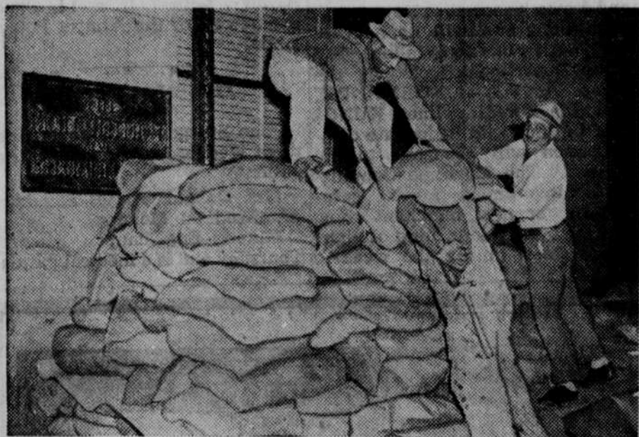
Following almost nightly air raid alarms and blackouts of San Francisco since the start of the war, the Pacific Telephone and Telegraph company has installed a sandbag barricade across the front of their building. Workmen are shown erecting the wall of sandbags, which will protect vital telephone equipment from possible enemy bombs.
