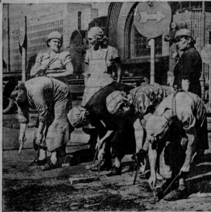
FINNISH WOMEN have had the privilege of voting since 1906 and through the years have assumed many tasks normally assigned to men in other countries. Here a group of them are laying paving stones in front of the new post office and station in Helsingfors, the nation's center of government.
