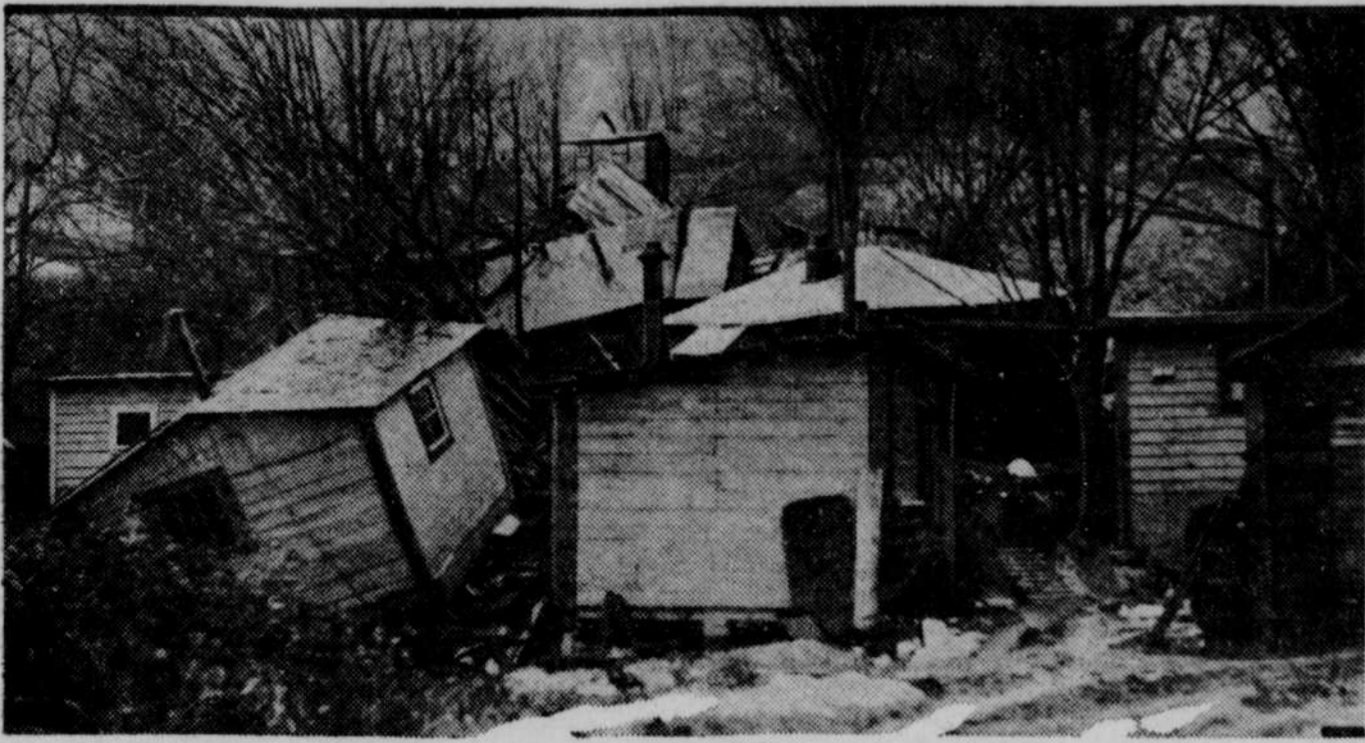
When a half dozen houses try to occupy the same building lot it's just too bad. The fast melting snow on Beacon Hill, Seattle, washed down over the sides of a colony of cliff dwellers and moved six or eight houses into one small space.
