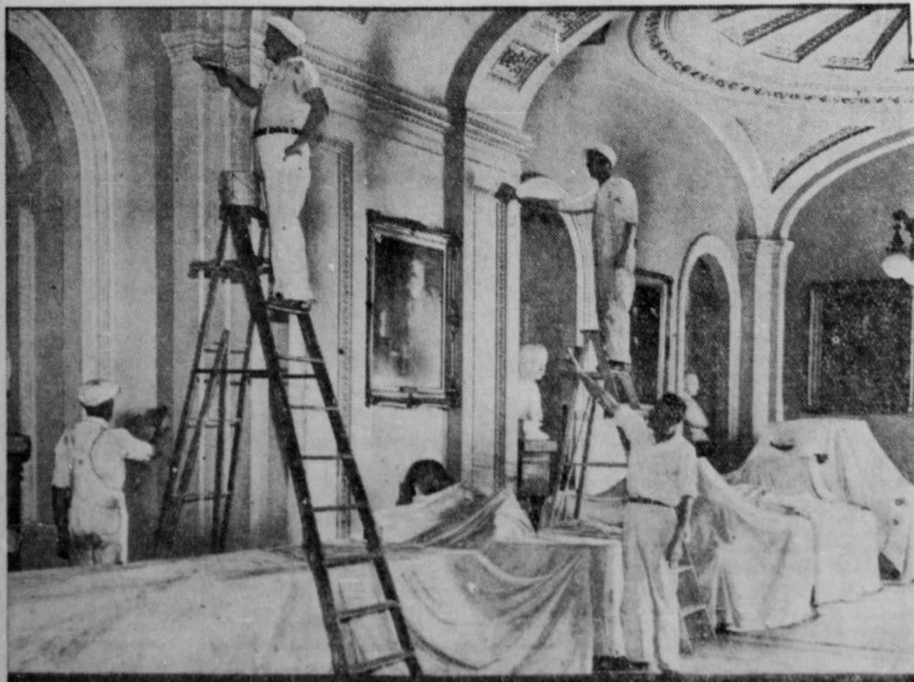
Painters are seen busily at work in the main corridor of the senate wing of the Capitol. A program of painting, redecorating, elevator installing, reconditioning of plumbing and general improvement such as has never been equaled since the British raid of 1814, has been under way. As a result it wouldn't be surprising if many congressmen fail to recognize the old place when—and if—they return.
