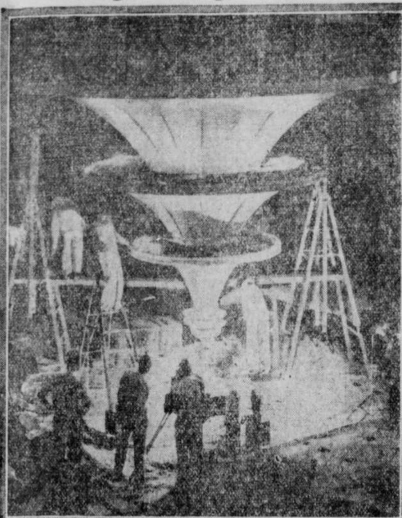
Weighing 6½ tons and measuring 25 feet in diameter, this giant chandelier, said to be the largest in the world, is being made ready for installation in the International Music Hall of Rockefeller City. An idea of the size of the big lamp may be gauged by comparison with that of the men working on it.
