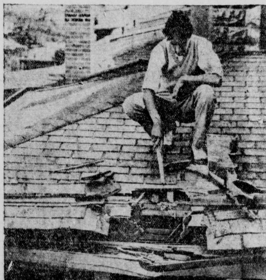
The hole to which this boy is pointing was made in the roof of a dwelling in Canarsie, L. I., by a 9-pound smoke bomb, dropped by a Naval Reserve "hell diver." The sea fliers were engaged in target bombing practice on Center Island when the accident occurred. It is believed a miscalculation in the use of the dropping device was to blame.
