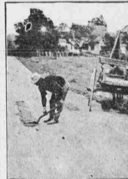
Repairing Road—Cheapest and Best Way is to Attend to Holes and Ruts While They Are Small.
