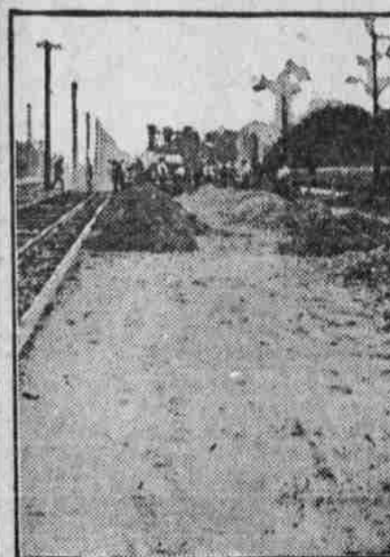
Sand and Gravel Piled on Subgrade Ready for Use on Experimental Concrete Road, Chevy Chase, Md.
