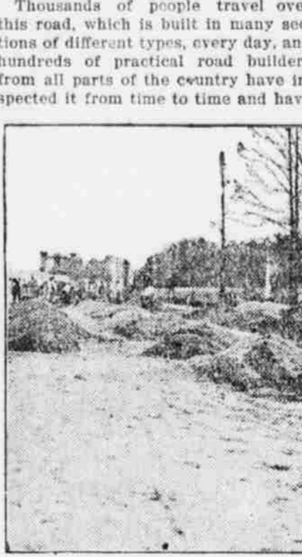
Sand and Gravel Piled on Subgrade Ready for Use, Experimental Concrete Road, Chevy Chase, Md.
