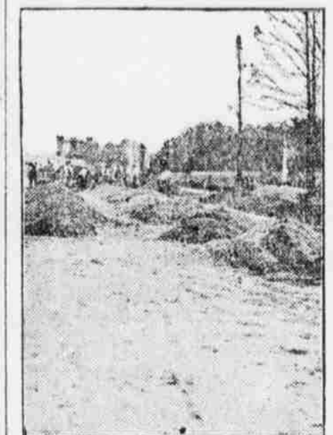
Sand and Gravel Piled on Subgrade Ready for Use, Experimental Concrete Road, Chevy Chase, Md.
