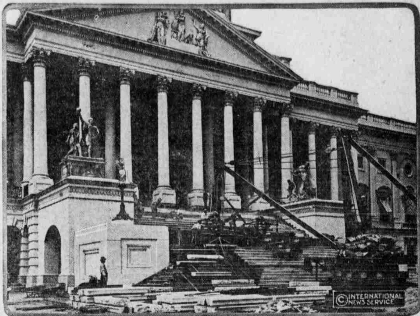
Workmen putting in new marble steps at the capitol at Washington to replace the old sandstone steps which time and the weather had rendered unsightly.
