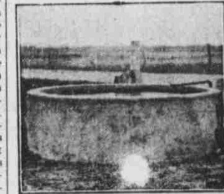
FIG. IV.—TANK—WILL NOT RUST OR ROT, so that they will not be cracked by ice in winter. After the forms are removed brush the inside of the tank with a paste of pure cement to prevent any leakage.
