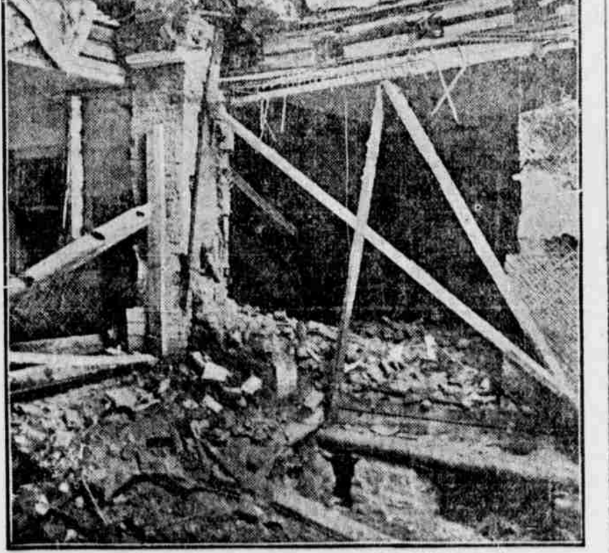
INSIDE OF THE VILLA AFTER THE EXPLOSION.
