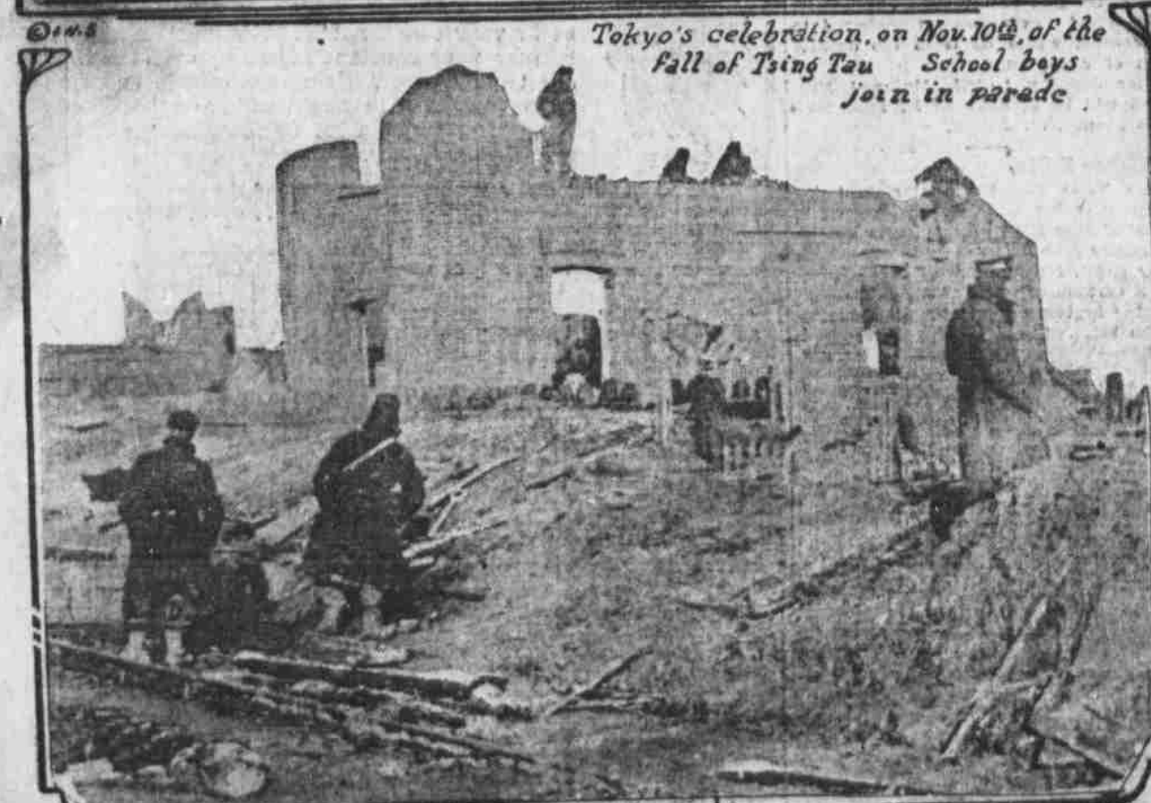
Belgians removing possible cover for the Germans by demolishing remnant of railway building at Perwyse
