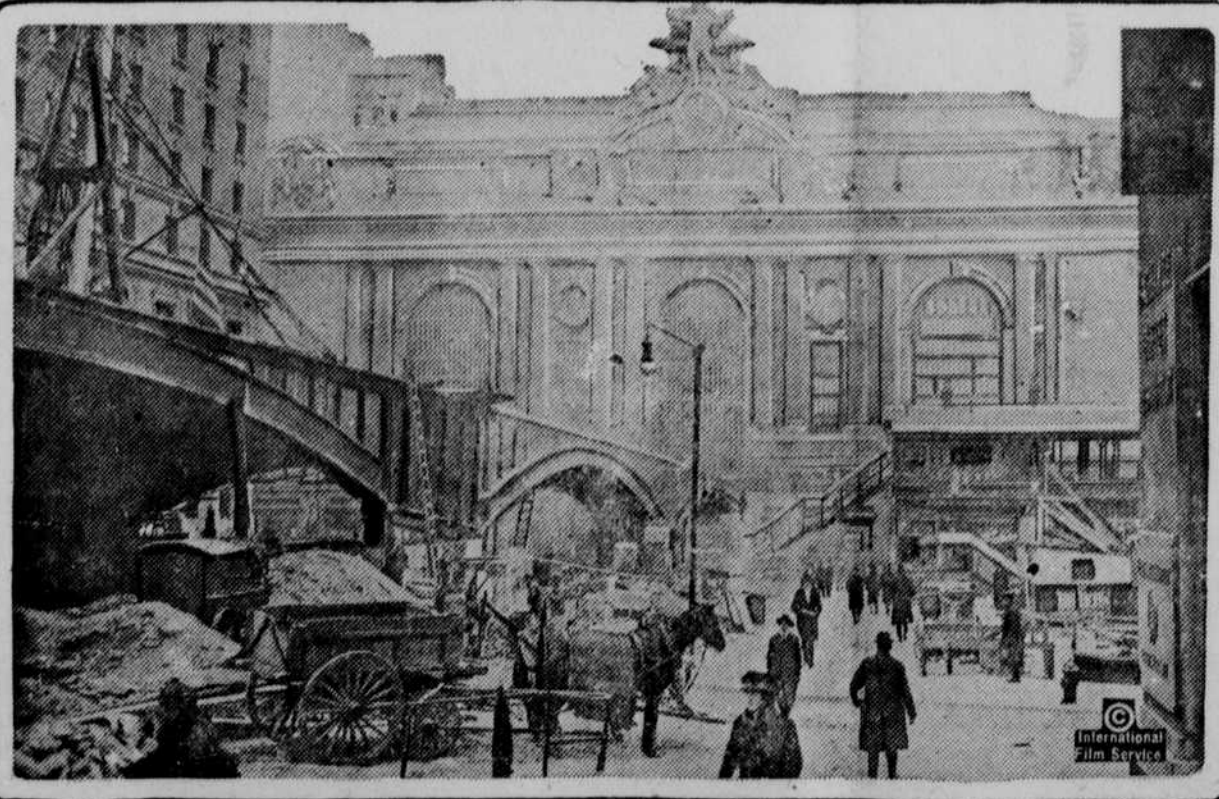
"Pershing square," New York city, so renamed in honor of our commander in France. The square faces the Grand Central terminal. The photograph shows the new runway into the terminal, which is now nearing completion.
