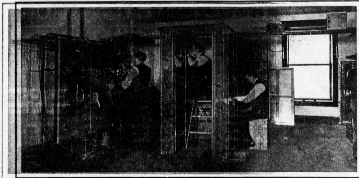
Power Board and Connection Switches
