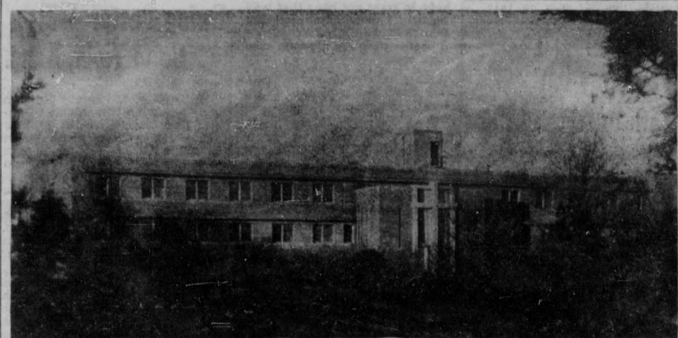
ST. ANTHONY'S NEARS FINISH . . . Workmen are in the home stretch on the new half-million dollar St. Anthony's hospital here. Plastering is being completed and interior painters will begin their work December 1. Within about a week the terrazzo floors will be laid in the corridors, entrances, 2 operating rooms and delivery room, and quarry tile will be placed in restrooms and shower stalls. Construction Superintendent Olaf Mathisen said this week that only miscellaneous concrete work remains to be done on stairways and landings. Already the heating plant is in operation on all 3 floors, the electricians are abreast with the plasterers and the laundry equipment goes in within 2 weeks, Mathisen said. Landscaping will not be done until later. In midsummer Mathisen estimated November 1 would be the finish date. Bricklayer labor problems and adverse weather caused considerable delays, he explained.
