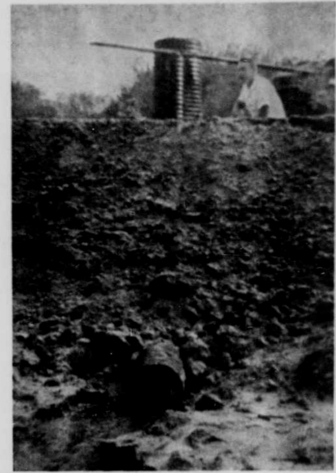
One of the dams built this year on Henry Walters place. Gene Schneider, part time conservation aid looking over installation of new type of tube. Small tube inlet takes water from lower part of pond. Water will be maintained at level of board where this tube empties into larger overflow. This design is especially recommended for ponds to be stocked with fish.
