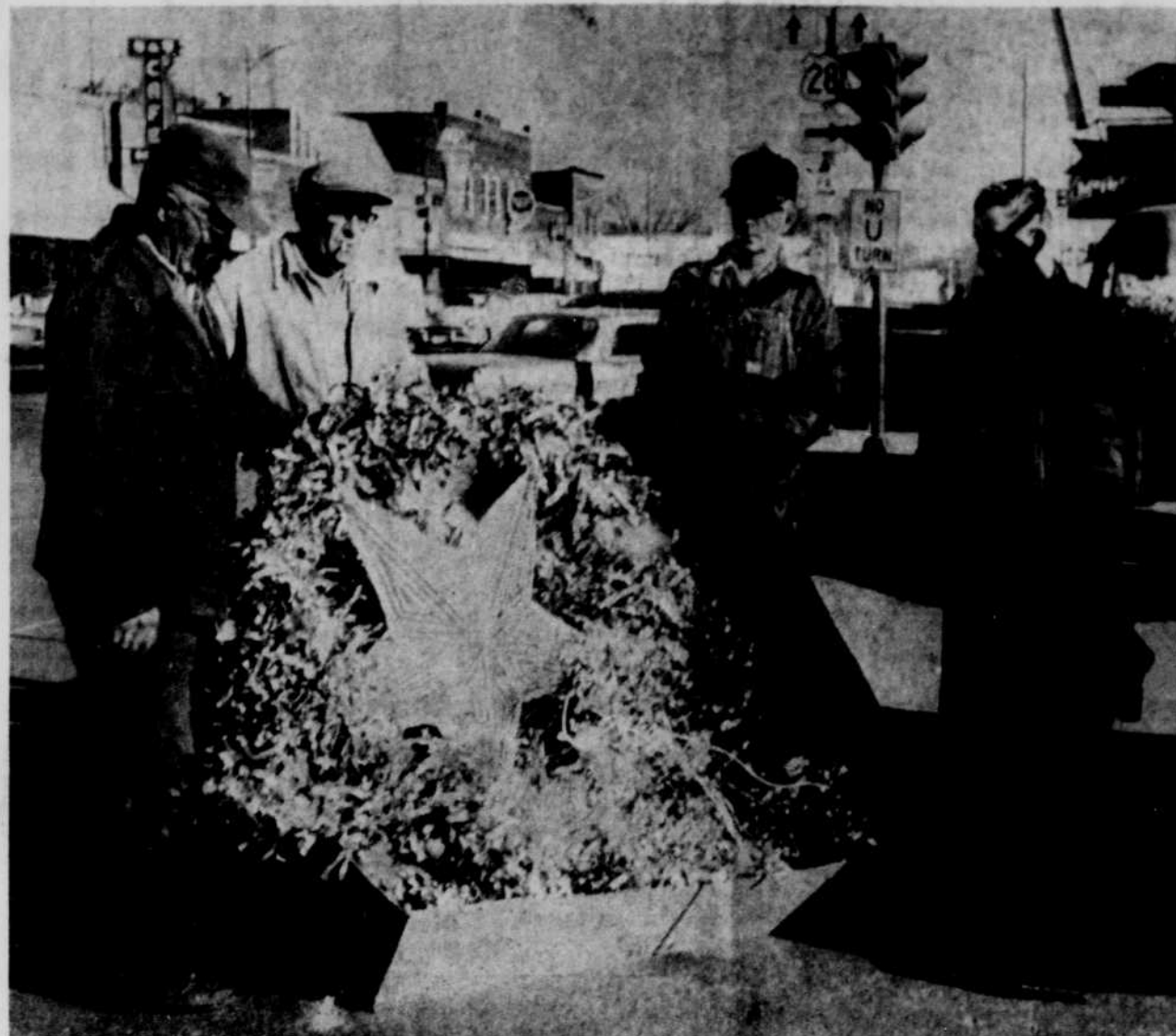
CHRISTMAS LIGHTS — City workmen, with an assist from Consumers Public Power District, have been busy erecting O'Neill's holiday lighting system. They are shown here as they prepare to raise one of the main ornaments at O'Neill's main intersection.
