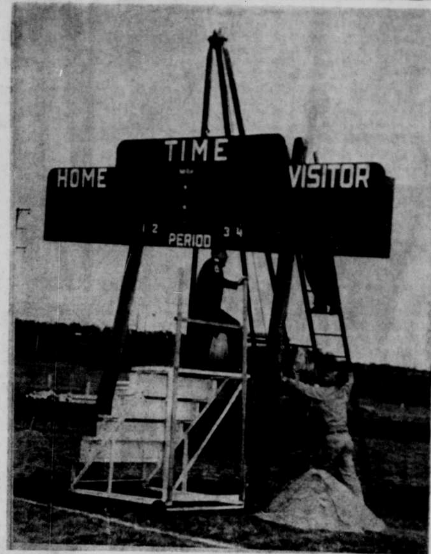
NEW SCOREBOARD — O'Neill's new football scoreboard was erected just in time for Friday night's game. Sgt. Cousins is shown here as he and workmen from REA hoist the board into place.
