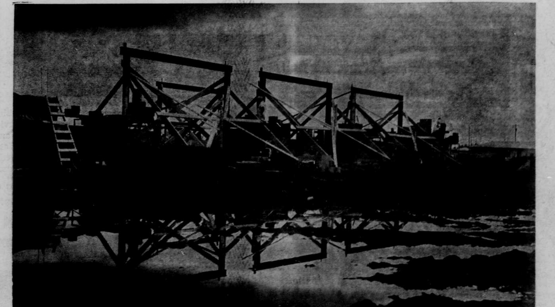
CONTINUED RAINS HAVE FAILED to have much effect on the construction of the O'Neill armory on North Fourth street. The north end of the building is shown here Tuesday morning with door beams reflected in water puddles as workmen hurry to cover fresh
