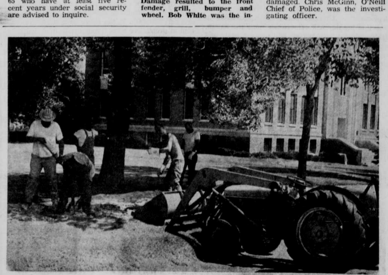
Workmen began the task Wednesday of replacing the sidewalk in front of the courthouse and the walk to the front entrance. This was one of the projects approved by the Board of Supervisors at their meeting Friday and Monday.
