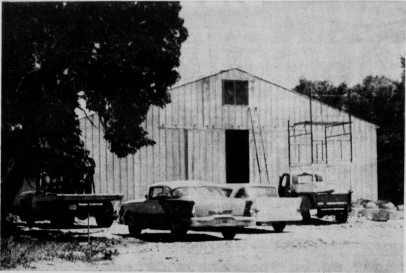
Ownership of the Page elevator passed into the hands of John Dienes of Orchard last fall. During the winter workmen repaired the building and gave it a complete coverage with aluminum siding. Tuesday work was completed on the new 50 by 140 ft. grain storage bin (shown above) having a capacity of 100,000 bushels. The original elevator was built in 1905 by Thomas Wade, whose son operated it in 1909. In 1928 Wallace French operated it for the Farmer's Union. A. G. Braddock took over as manager in 1939. Other owners have been Albert Ellis, Ed Hubbard, Jack Weber, Dave Deaver, Don McKamy, Charles Sorenson and the Meuret Grain Co. Now the elevator will again be open for competitive business.
