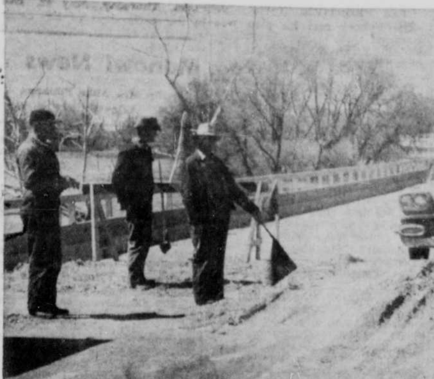
Highway crew members watch the Elkhorn river bridge east of O'Neill. Shown above are David McClintok and Myrl Cady of Ainsworth and Paul Biner, Inman, with the flag. Frontier photo and engraving.
