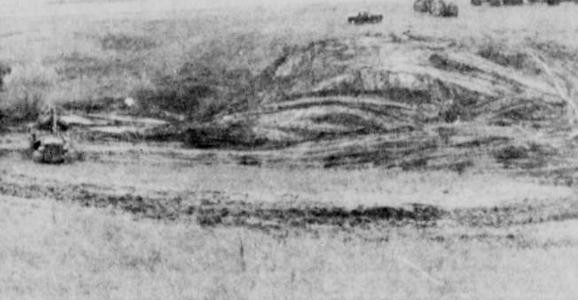
Dam under construction on Harvey Krugman farm. This was a part of Mr. Krugman's Great Plains contract. Smith and Son of Verdigris, contractor.
