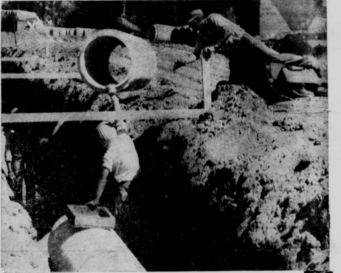
Workmen lower large sections of concrete culvert on north Second street in preparation for the paving crew of 50 to 60 men. The Frontier Photo and Engraving.
