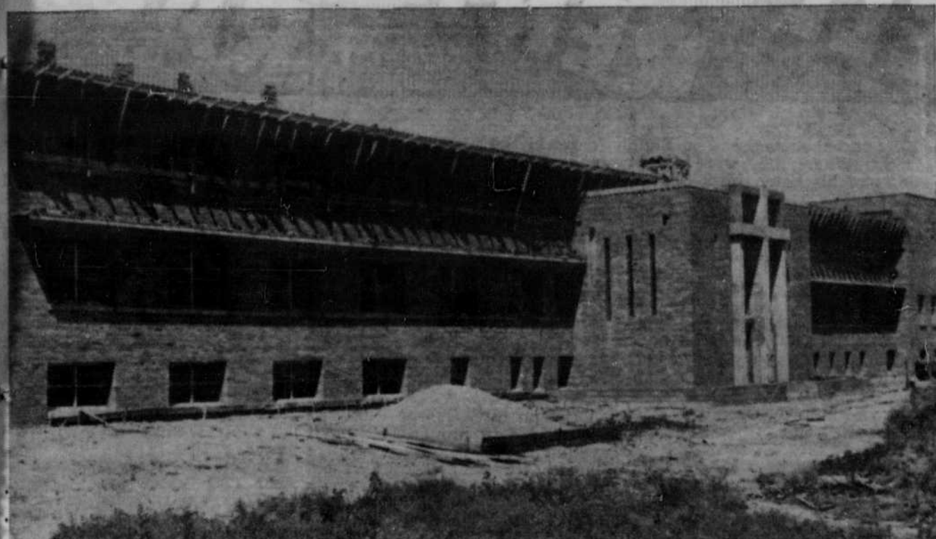
ST. ANTHONY'S PROGRESSES . . . October 1 has been fixed as the finish date for the near half-million-dollar St. Anthony's hospital under construction here. This week the roof is being poured. Olof Mathisen, foreman of the Busboom & Rah Construction Co., says completion of the roof will be an important step because finishing
