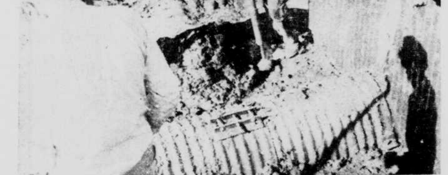
DAM BUILDING is more than just moving dirt with big machinery. Where tubes are needed much hand labor is required. Diaphragms are installed and the dirt is back-filled and tamped with pneumatic hammer. Operating the hammer is Bill Mittes, contractor from Royal furging the construction of a dam for Norman Saltz, east of Page.
