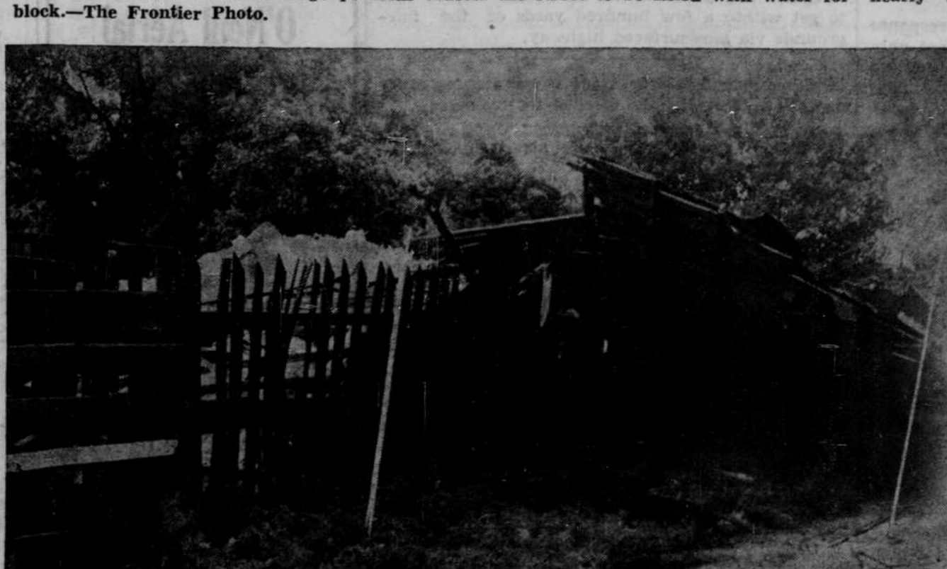
This is a view of the demolished Ryan hay barn, one-half block west of the J. B. Ryan company office building. This was the only building badly damaged by Tuesday's wind, which was described by several eye-witnesses as a small twister.—The Frontier Photo.
