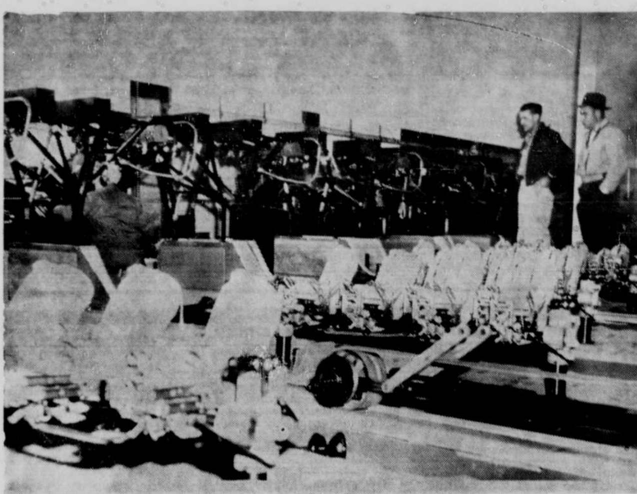
This maze of equipment being installed at the "business end" of the Ten Pin Bowling Alleys might have been a rocket launching mechanism as far as the photographer is concerned. The last of eight automatic pin setters is being hoisted into position (left center) while J. W. Rockwell (extreme right), one of the owners, looks on. The alleys will open for business Saturday.—The Frontier Photo.
