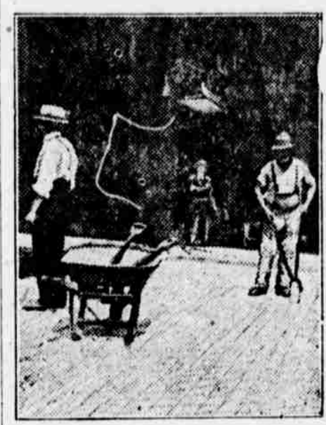
Granite Blocks Laid and Rammed—Maintenance Cost of This Kind of Pavement is Less Than That of Any Other Kind.
