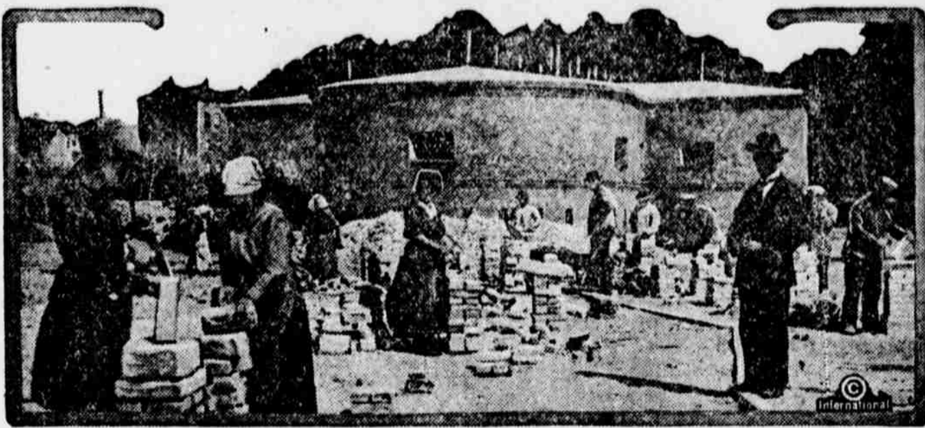
The fort of Spandau, in accordance with the terms dictated by the armistice, is being demolished by the Germans. Women are doing most of the work, the stones when loosened being piled up with care for later use in the erection of dwellings. Spandau is the famous treasure house of Germany. In this great fort were kept tons of gold collected for just such a war as has been lately declared ended.
