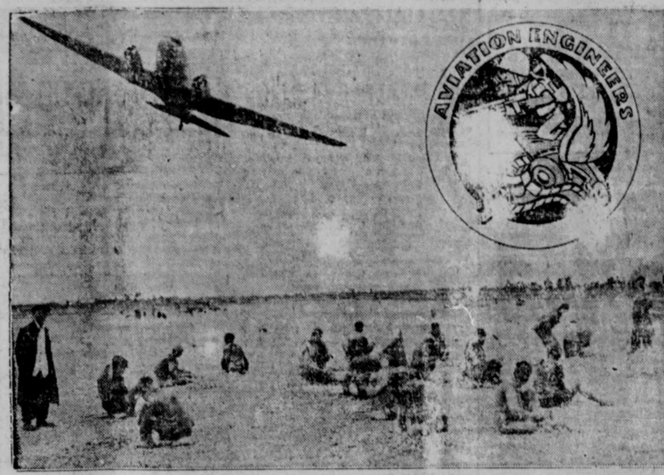
Released by U. S. War Department Bureau of Public Relations. AAF AIR FIELD IN CHINA—Willing Chinese labor, working under methods of 1,000 years ago nevertheless soon aviation engineers direct the job. Inset, "bucking bulldozer," unofficial insignia of the Aviation Engineers. (Army Air Forces photo).
