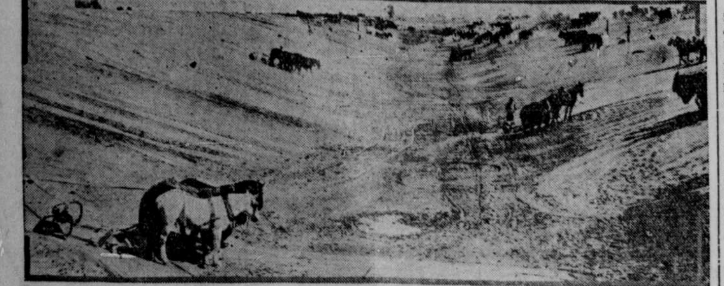
One hundred four-horse teams are here busy on one section of the All-American canal which will replace the main now serving California's Imperial Valley. The new canal will have a width of 232 feet, a depth of 21 feet and will carry the water of the Colorado river 80 miles across the valley for irrigation purposes. The men and teams shown in the photograph above have moved more than 1,000,000 yards of earth with their Fresno scrapers.
