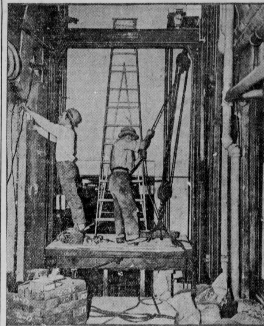
Workmen are shown installing new high-speed elevators in the Capitol building in Washington. The old ones were too slow for the congressmen.
