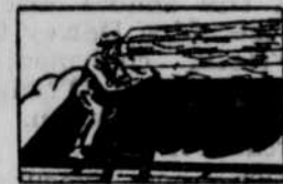
THE ROOF is thoroughly examined and old shingles removed if necessary and desired.
