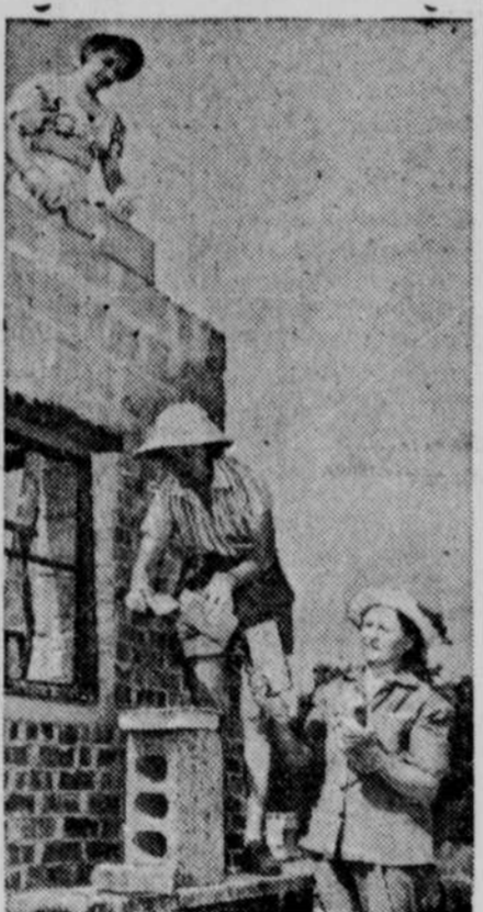
THIS IS THE HOUSE! . . . Out at Lemont, Ill., a house is rising which is different than the house that Jack built in the nursery rhyme, because much of the work is being done by a couple of Janes. Mrs. Joseph Gurski, center, is laying brick on the new family home, assisted by willing friends.
