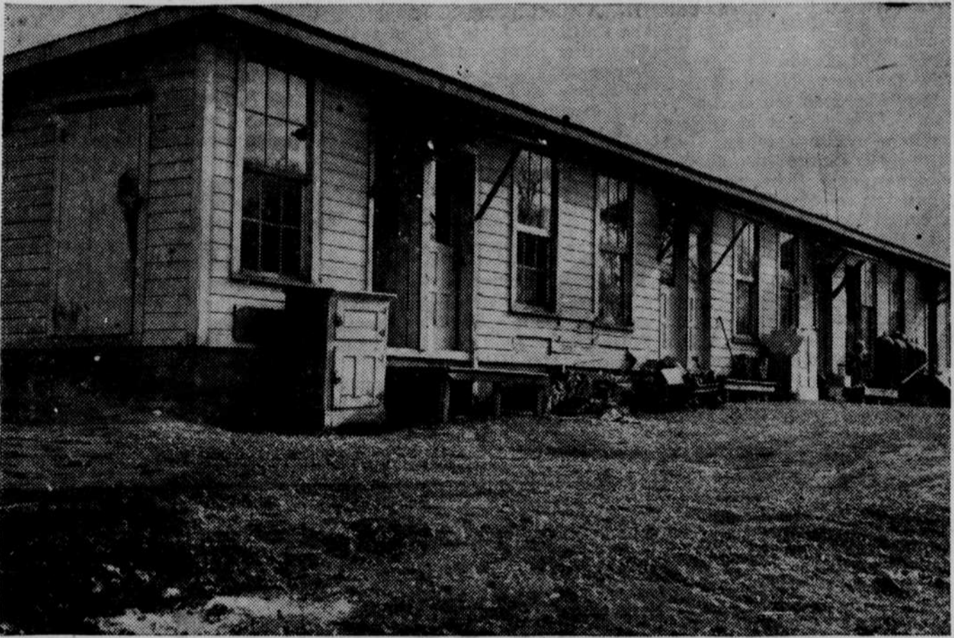
HIGH COST OF LIVING IN A CHICKEN HOUSE . . . A few weeks ago this was a chicken coop on the farm of Herbert Studebaker, Waterloo, Iowa. Today it is converted into eight one-room kitchenette apartments, with a utility room for use of all tenants. There were more takers at $52.50 a room per month, than the Studebakers could handle on their poultry farm. More revenue from renting than raising chickens!
