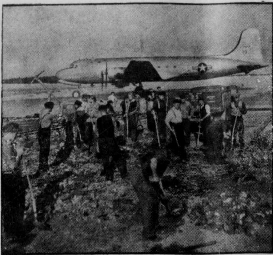
BERLIN AIRLIFT GETS A BOOST . . . Gatow airfield in the British sector in Berlin is being enlarged to better handle Allied planes flying the airlift. While some 400 planes bring in almost 3000 tons of food and coal daily, work continues at top speed to expand airport facilities before winter sets in. Here, German laborers lay a taxi strip foundation while a C-47 lands in the background.
