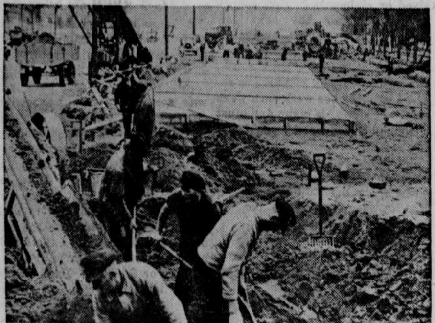
Construction work goes rapidly on the new broad highway that will bisect Berlin from west to east and is a part of the vast roadbuilding program undertaken by Hitler. In 1938 a total of 1,864 miles were added to the country's system of express motor highways.
