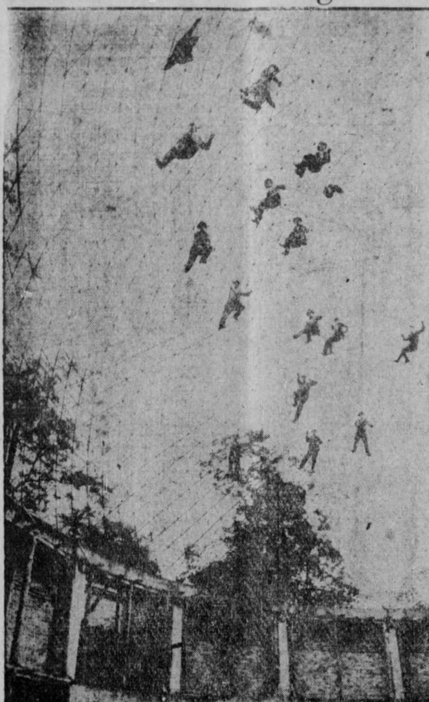
These workmen constructing wire framework as a base for a dome of a huge astronomical observatory at Berlin, Germany, look as hapless as flies entangled in a great spider's web. Each intersection is knotted with extreme care.
