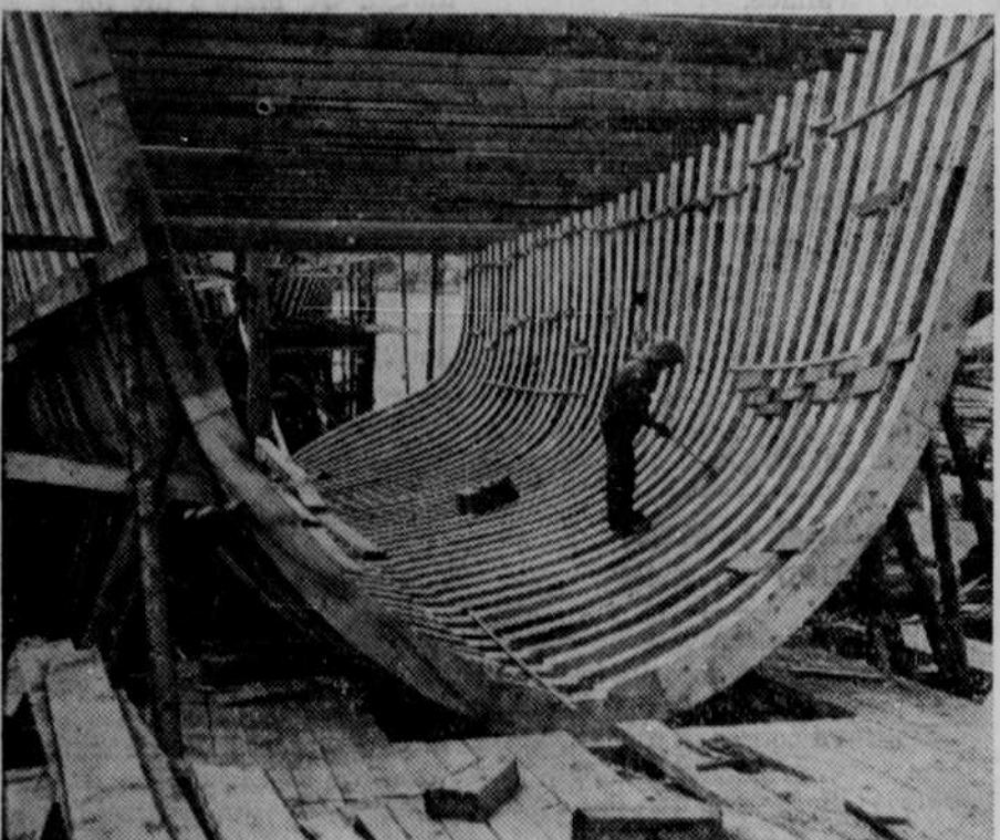
Old-timer Ray Rubshaw is working inside the framework of a hull under construction. He is dubbing or smoothing out and lining up the ribs for planking, using an adz.
