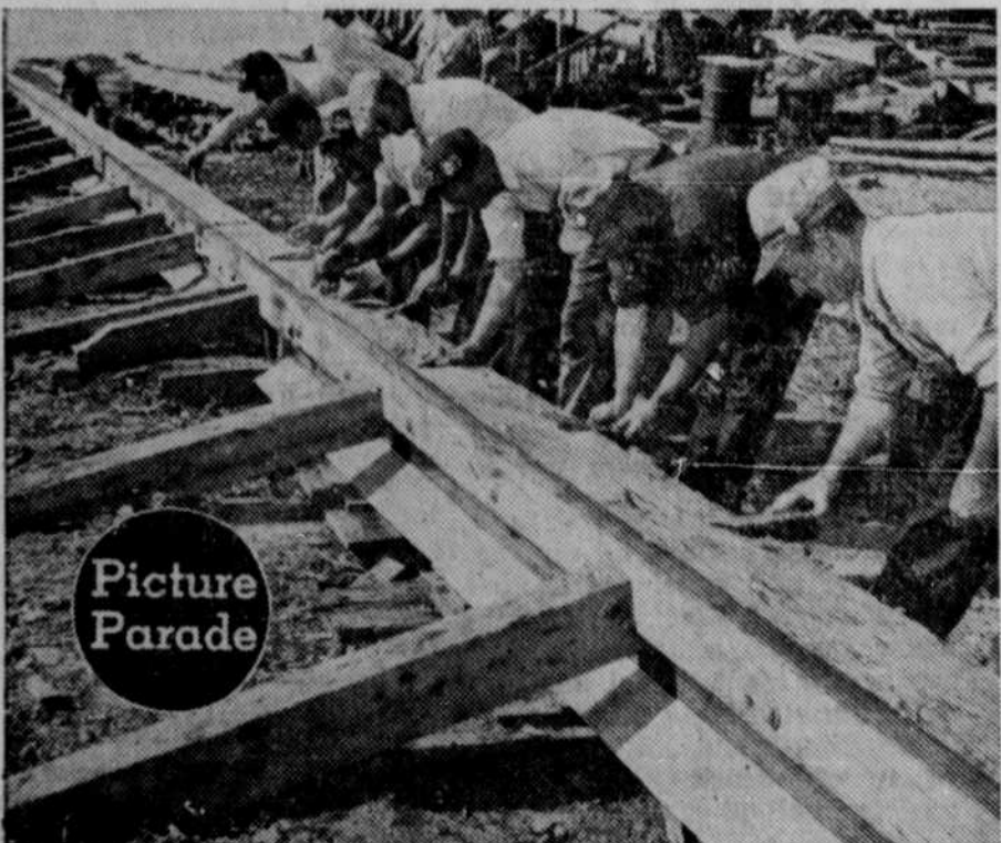
Greasing the skids before launching a completed wooden ship. Pounds and pounds of grease are smeared on the skid to make the slide of the new craft easy and to counteract friction.
